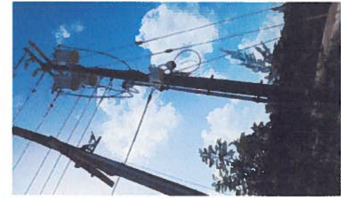
Electrical Mains Connected
